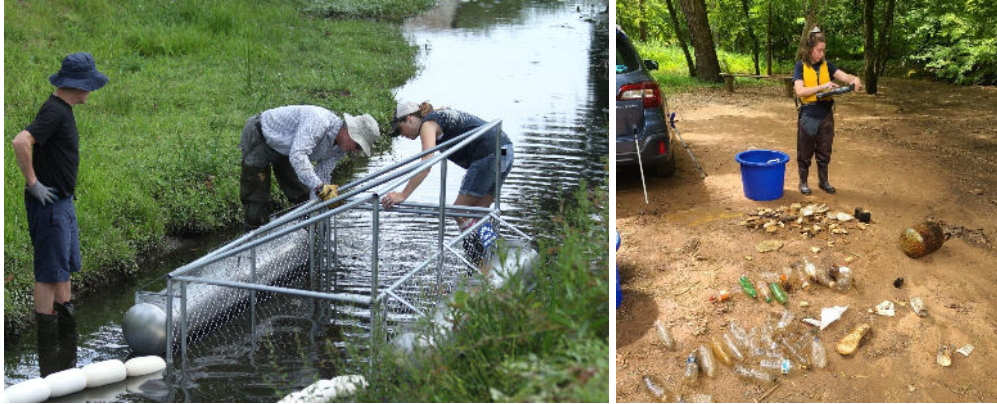
Figure 2: Left: Trash trap installation in Jacks Creek, Washington, NC. Right: Catawba Riverkeeper volunteer conducting trash audit.
